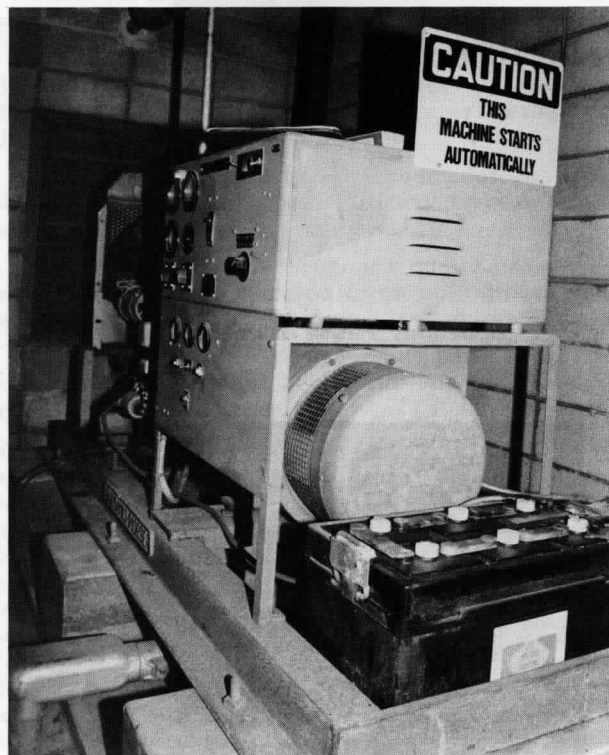
Figure 4-7(b) Emergency standby electric power generator.
